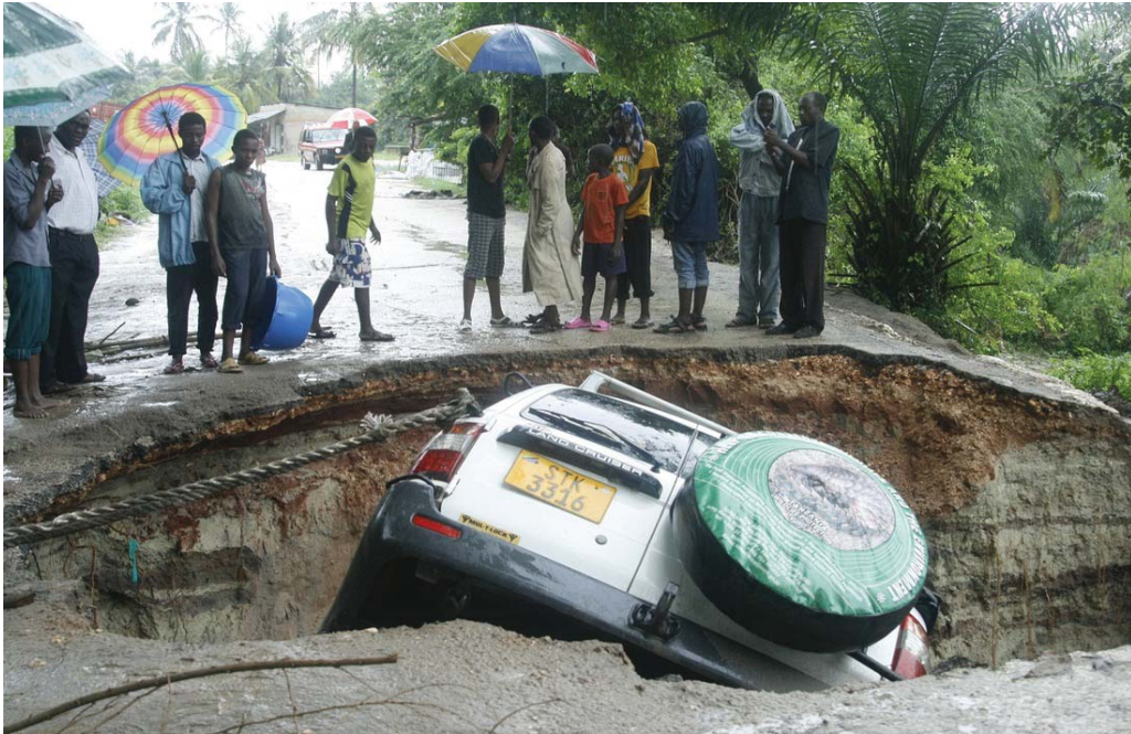
Figure 11: Road destruction by floods at Tandale Mtogole, 2011
